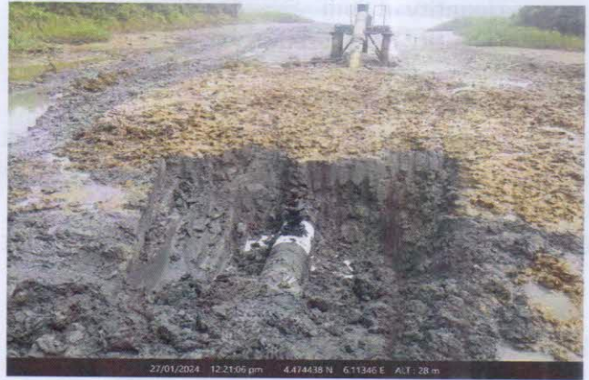
Incident point with 6" Valve Installed
